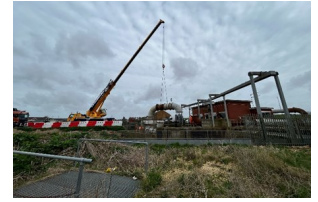
Trusthorpe Pumping Station
